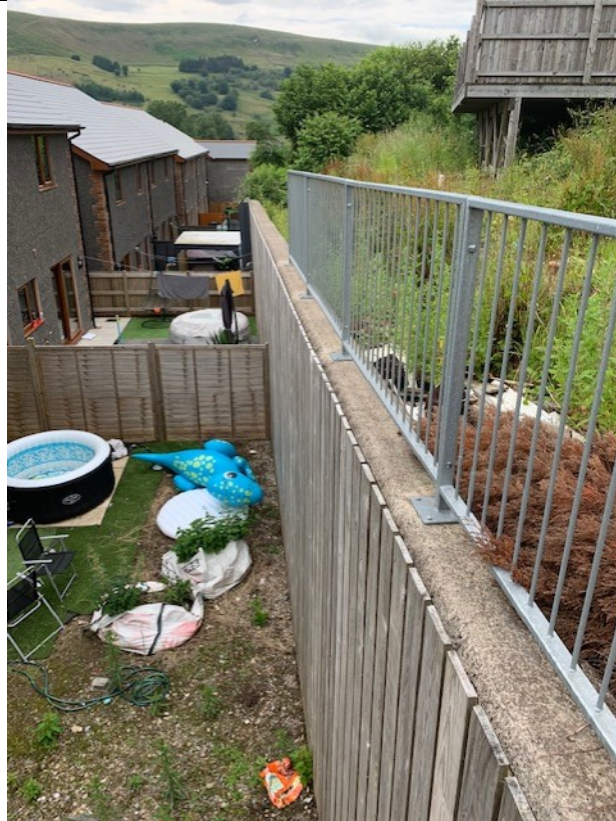
Photograph 13: showing the large retaining wall faced with timber boarding provided to the rear of properties 4-7 Rhos Yr Ysgol
