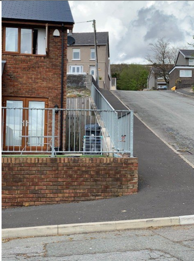
Photograph 7: showing eastern boundary with a mass concrete retaining wall at lower level topped by galvanised railings.
